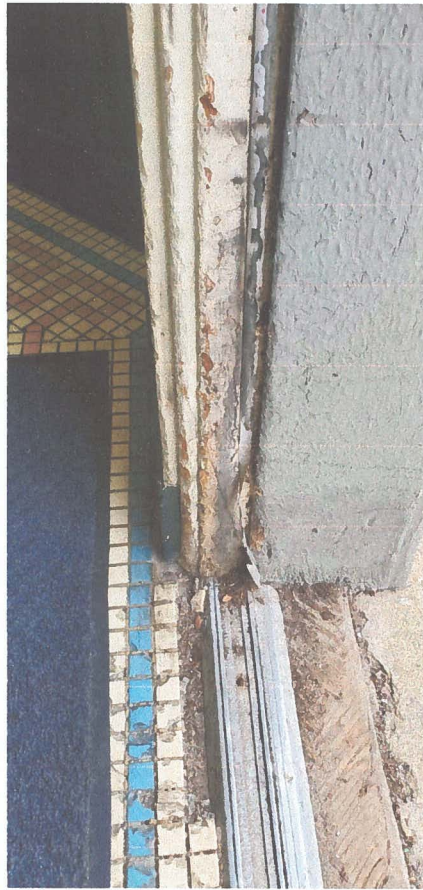
15 E. door frame is deteriorated, as is threshold. Does not seal well.
