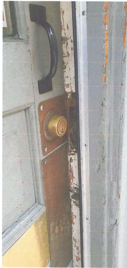
15 E. back door frame is deteriorated; door does not close properly.
