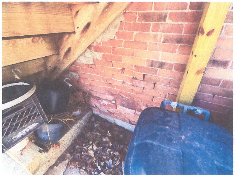
Damage brick to be repaired
