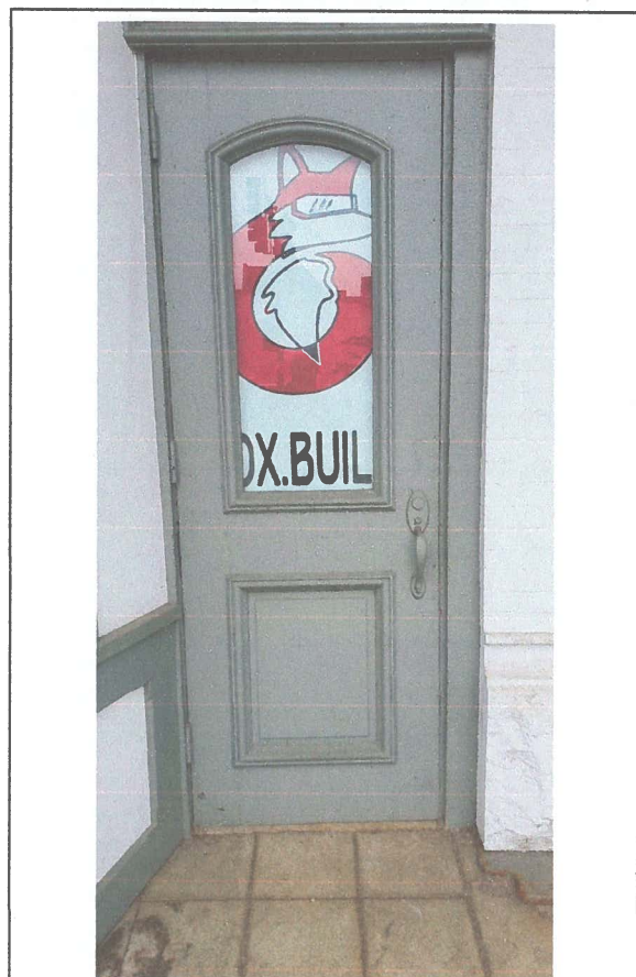
13 E. Main Door. Does not open from outside. Brass is painted over.
