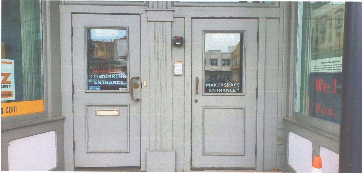
The 1 st and 2 nd floor doors at 11 E. Main. St. The mail slot is bent on the left door and the brass has deteriorated on all the brass parts. Neither closes tightly.
