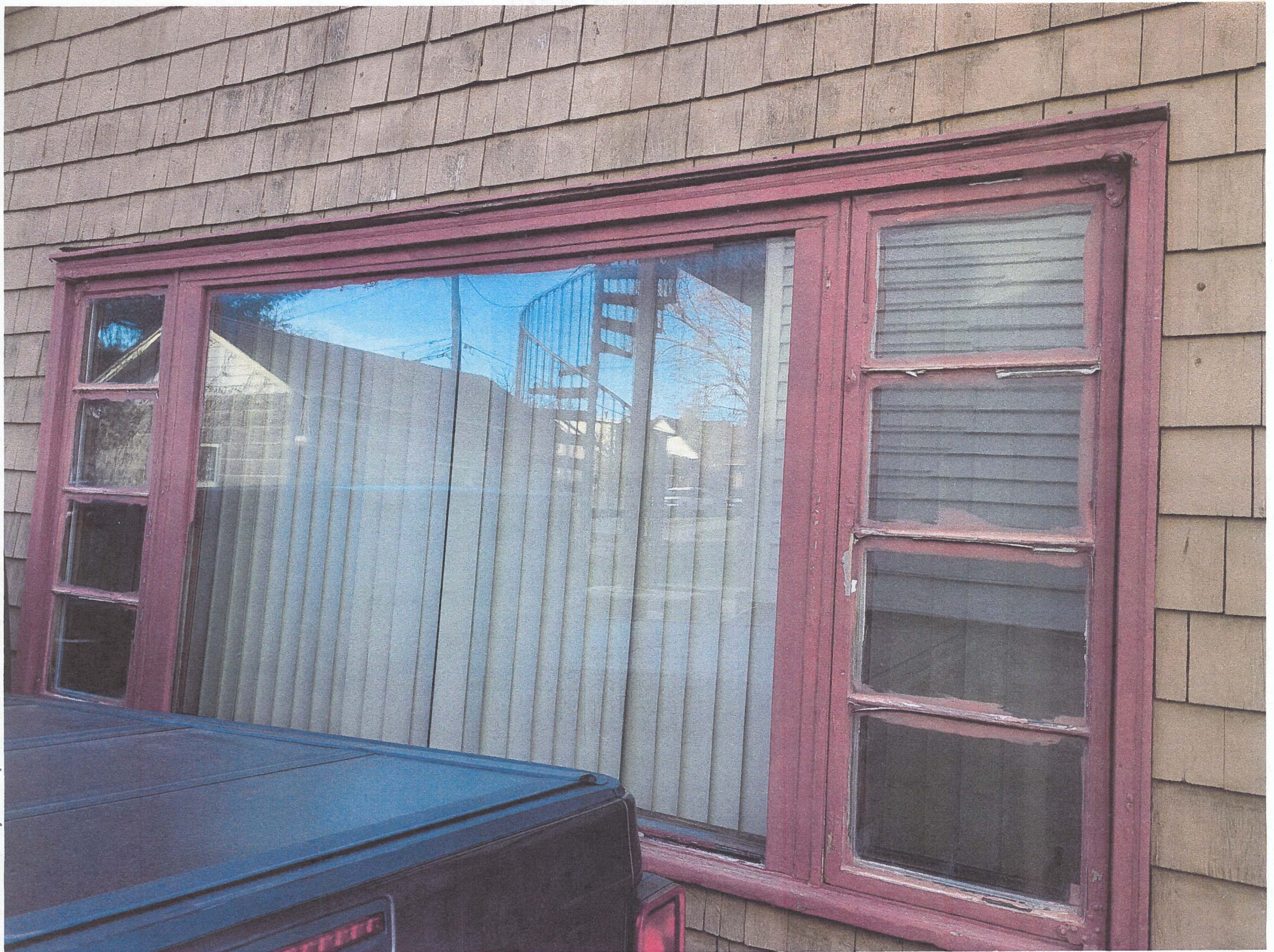
EAST WINDOW TO BE REPLACED
