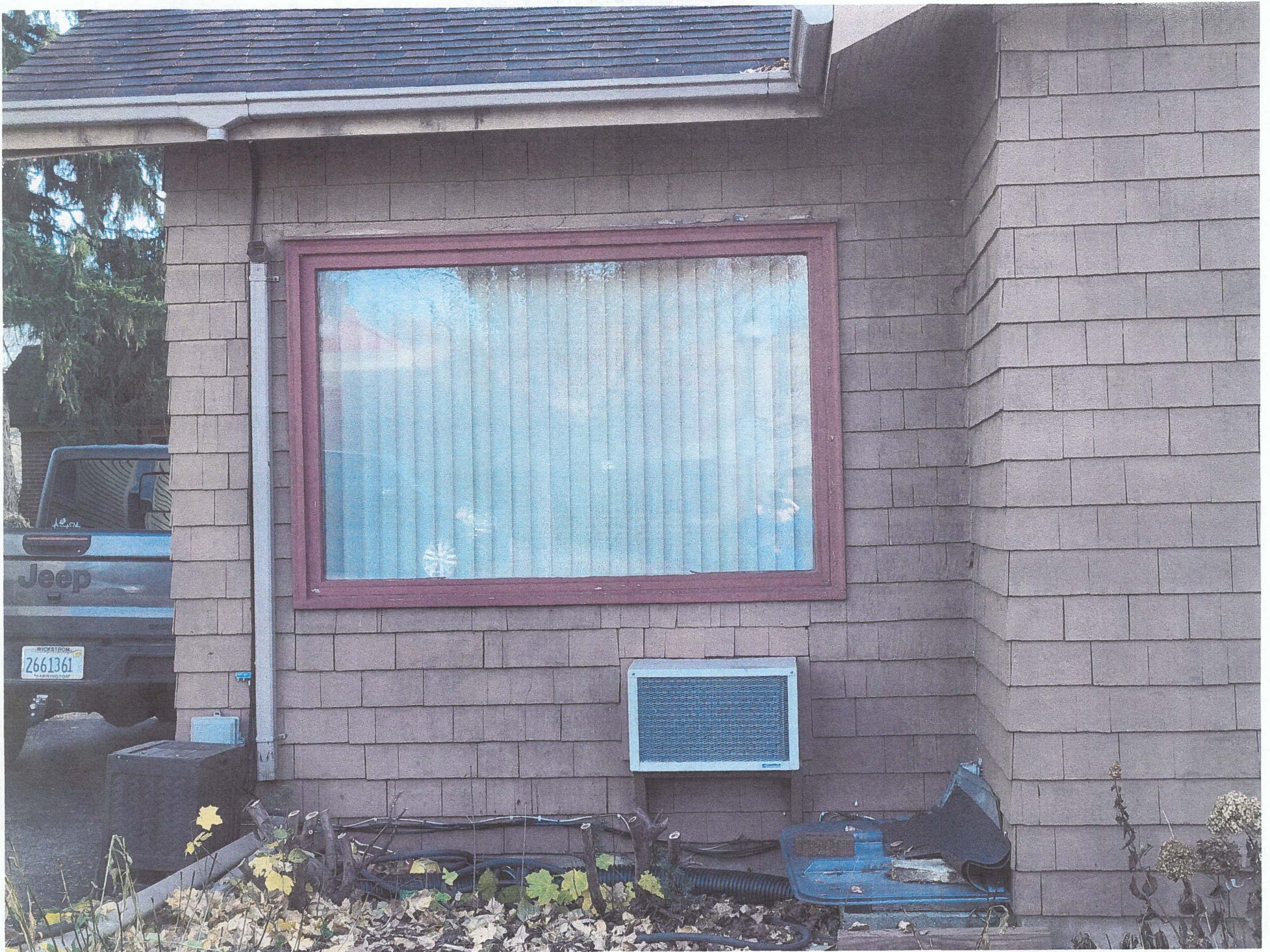
NORTH WINDOW TO BE REPLACED
