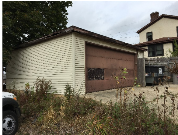
Detached Garage in poor condition
