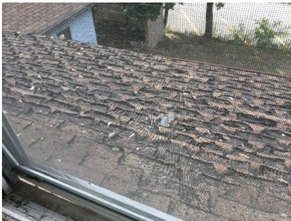
Shingles are curling due to extreme deterioration
