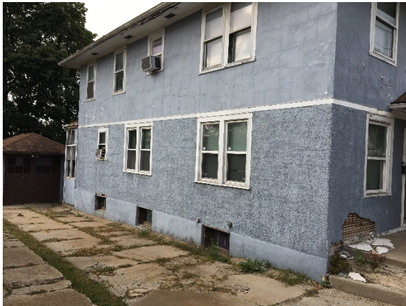
Driveway, stucco, soffit all in poor condition
