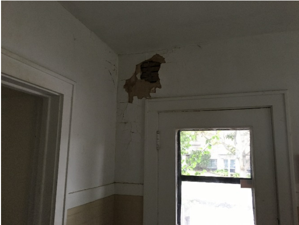
Interior stucco peeling
