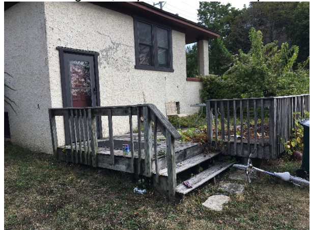
Deck overgrown and is unsafe to walk on
