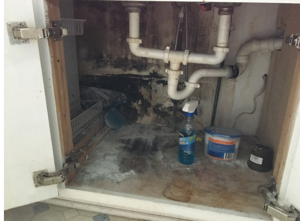
Mold and rot under kitchen sink
