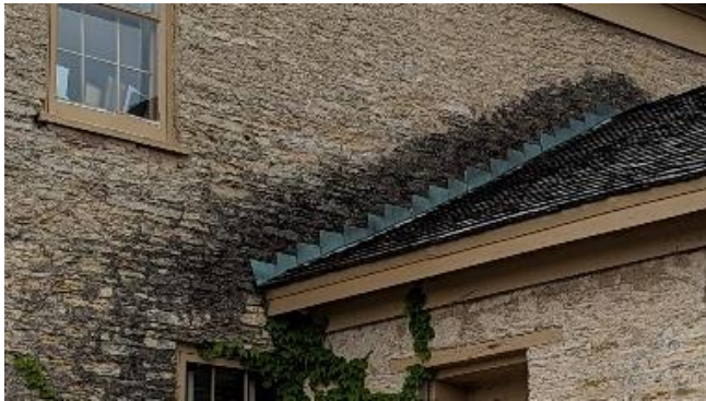
Damage to limestone on north façade
