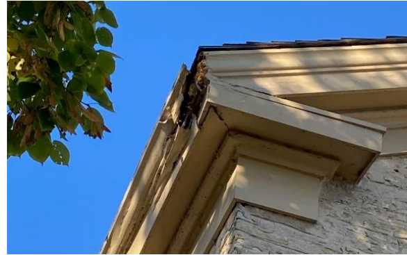
Damage to south crown molding, fascia, and soffit
