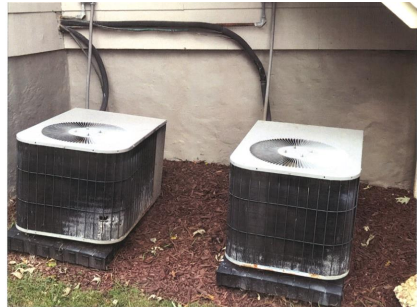
Separate Central Air Conditioning Units
