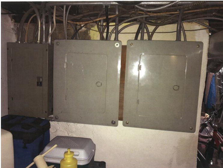
Separate Circuit Breaker Boxes for Each Unit
