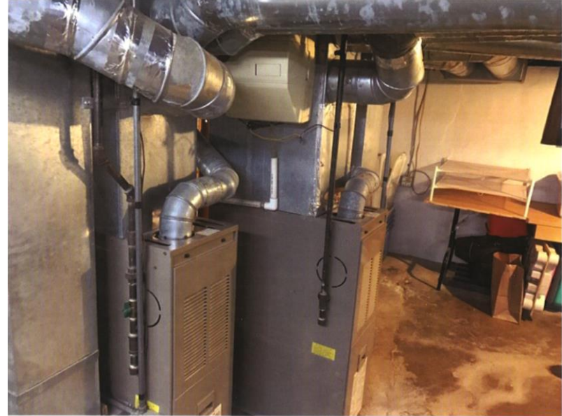
Separate Furnaces For Each Unit
