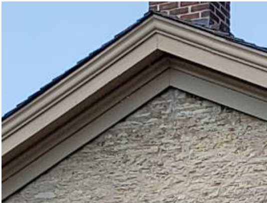
Deteriorated trim, prior to removal.
