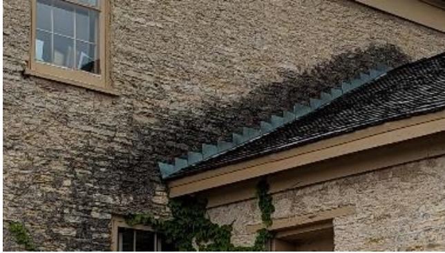
Damage to limestone on north façade
