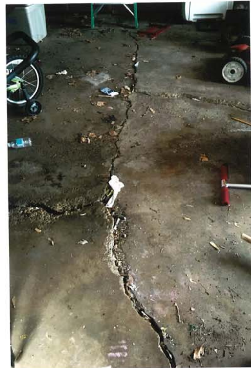
Cracks go E/W ↑
