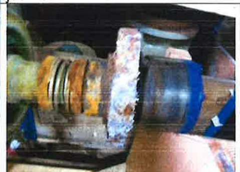
Mechanical seal in very poor condition
