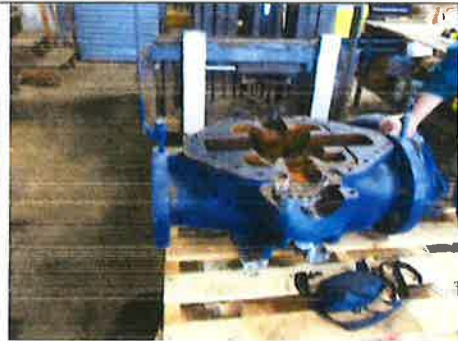
Booster A in Layne shop
