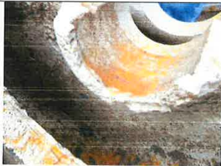
Extreme pitting and erosion at seal journals.
