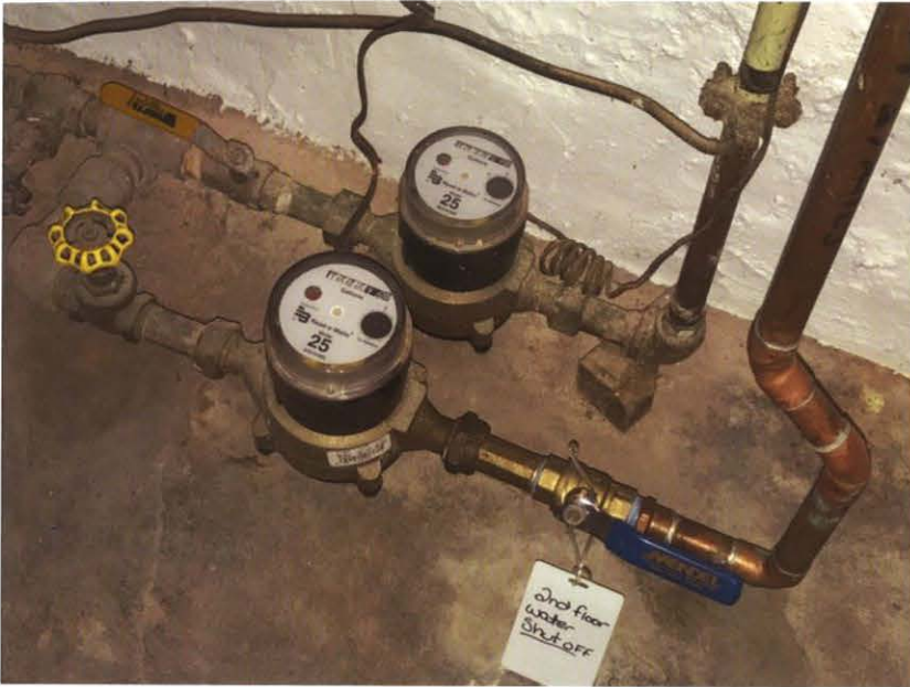
Separate Water Meters For Each Unit
