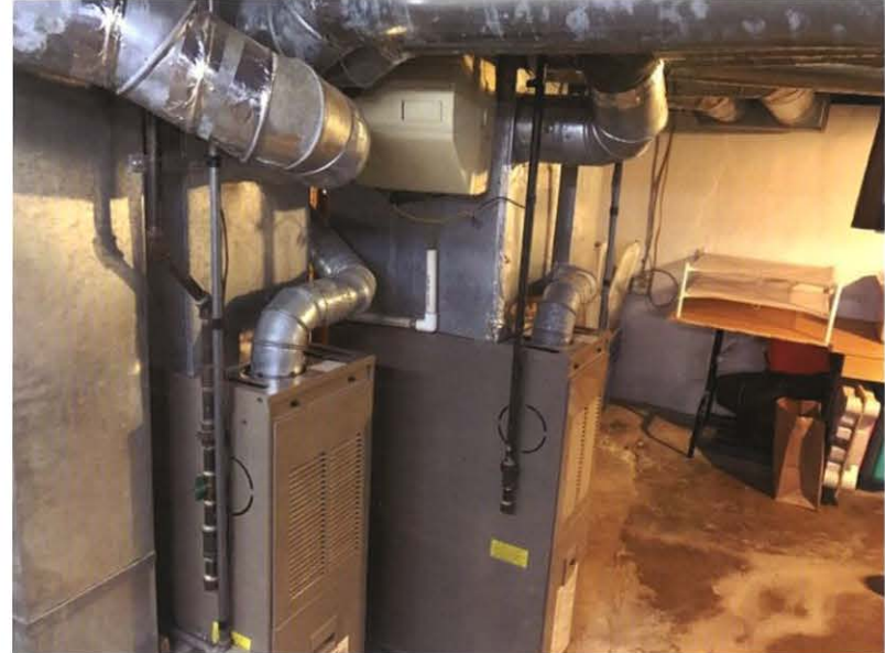
Separate Furnaces For Each Unit
