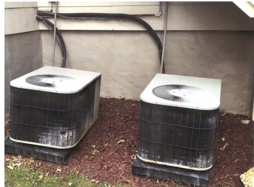
Separate Central Air Conditioning Units
