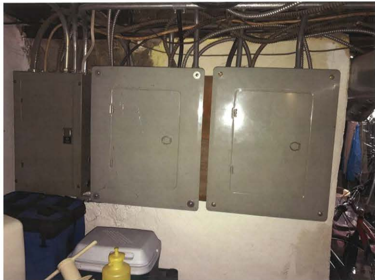
Separate Circuit Breaker Boxes for Each Unit
