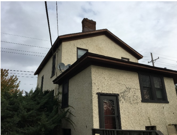
Rear of home, chimney missing bricks, stucco peeling.
