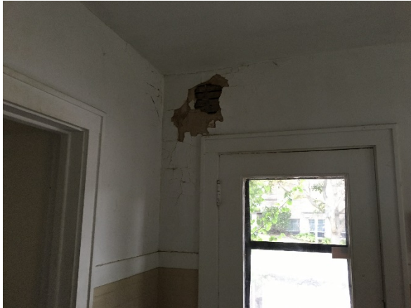
Interior stucco peeling
