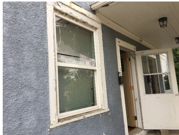
Broken front window
