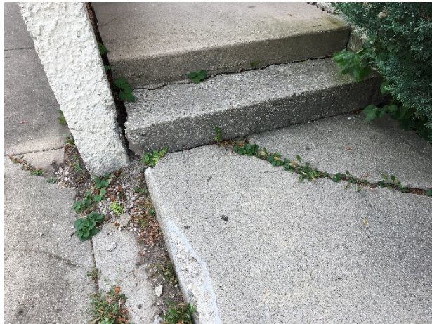
Front wall is falling over, steps and sidewalks in poor condition
