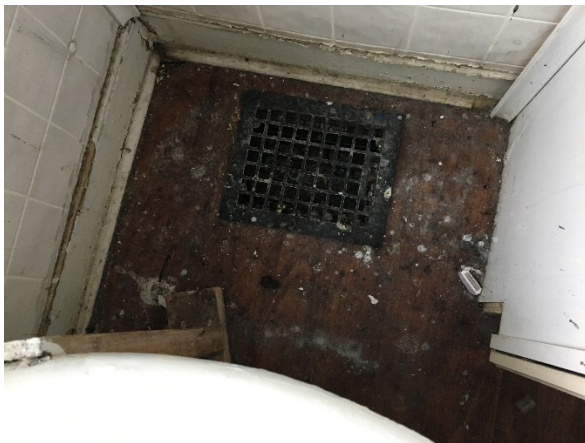
Mold in bathroom, likely inside duct work also
