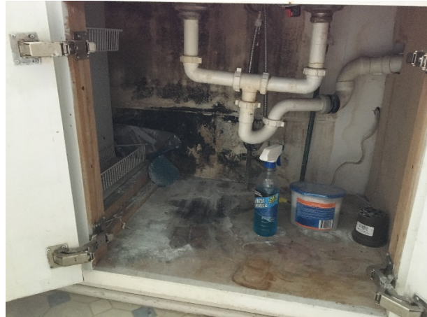
Mold and rot under kitchen sink
