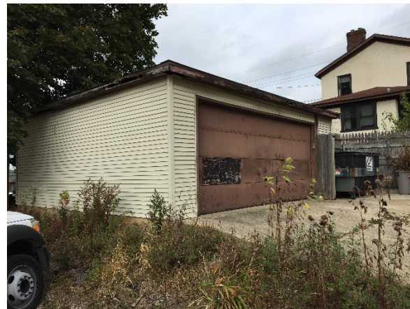
Detached Garage in poor condition
