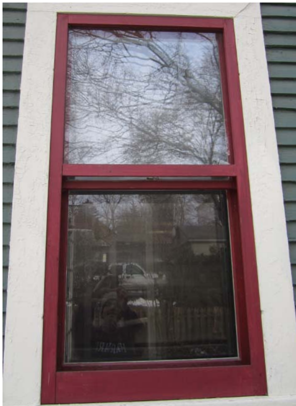
Some windows have broken wooden storm windows.
