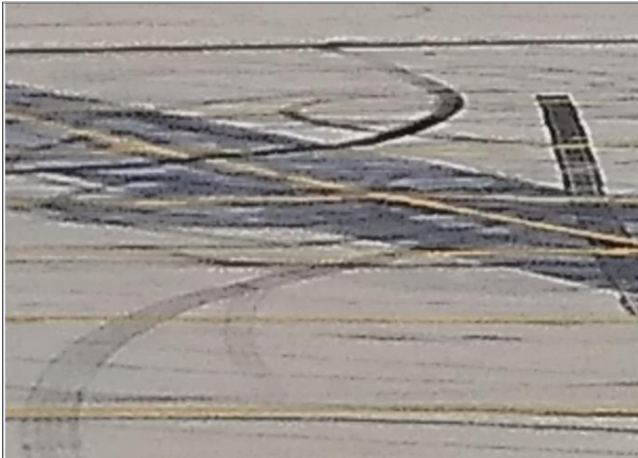
Figure 9: Skid Marks Due to Joyriding on Top Floor in Parking Garage
